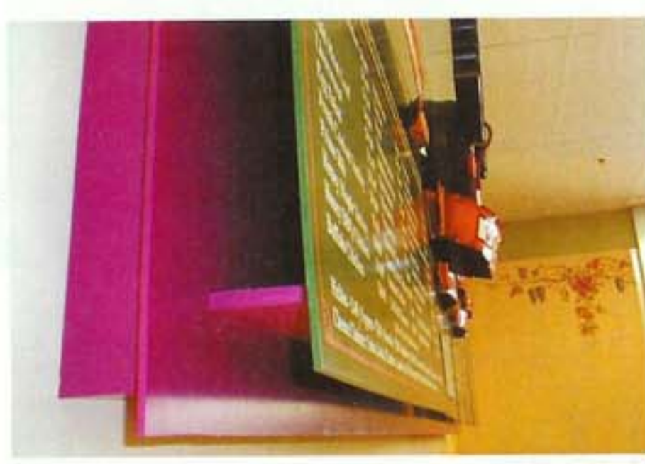
Ron and his assistant, Fernando Ocampo, created a frame using PVC, and affixed it to the signface using Weld-On cement, L brackets, double-sided tape and panhead screws.
